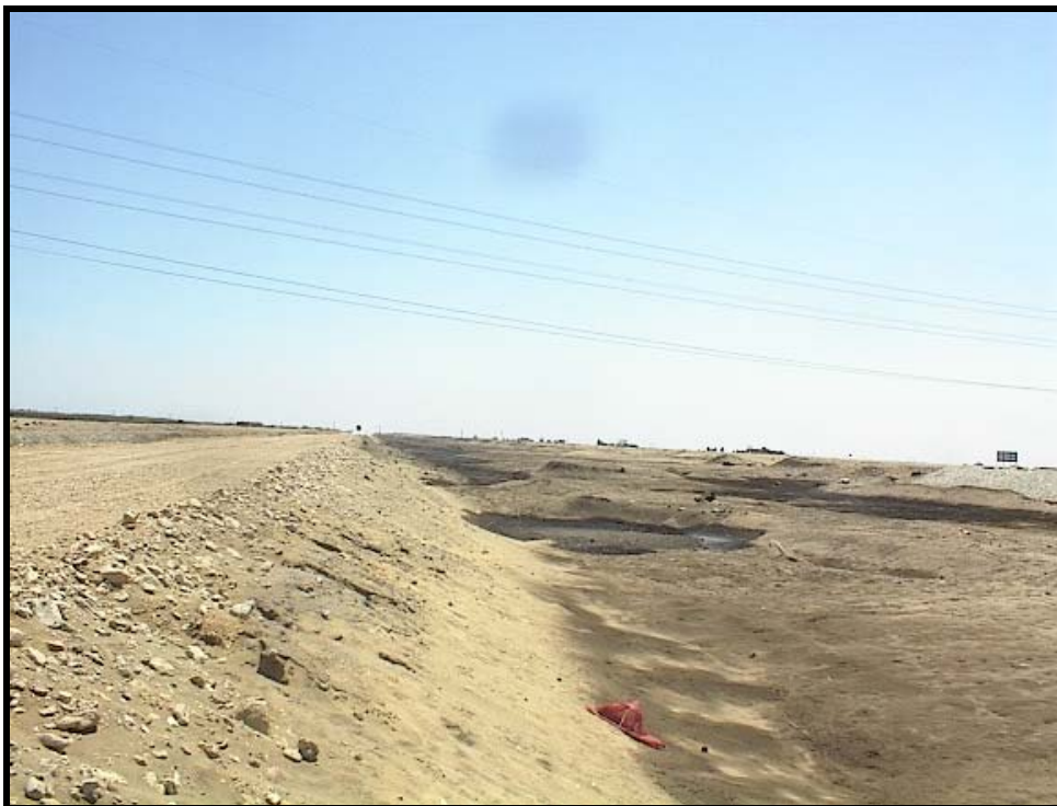
Photos 6&7 “The proposed pipeline route parallel to El-Sheikh Gaber canal for about 18 km “
