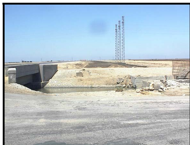
Photos 4&5 "proposed crossing location of El- Qantara Port Foad road and El-Sheikh Gaber canal"
