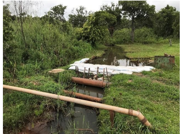
Figure 1 – General view of weir and area u/s, viewed from the road bridge, d/s
