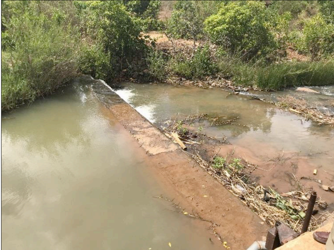
Figure 1.2: Existing low concrete weir at Ekwendeni as viewed from the right bank
