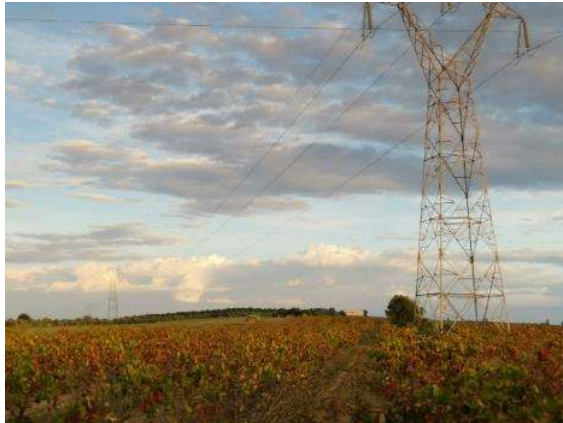
A tower (OHL 90 kV) installed in a vineyard near Menzel Bouzelfa Nord (Nabeul)
