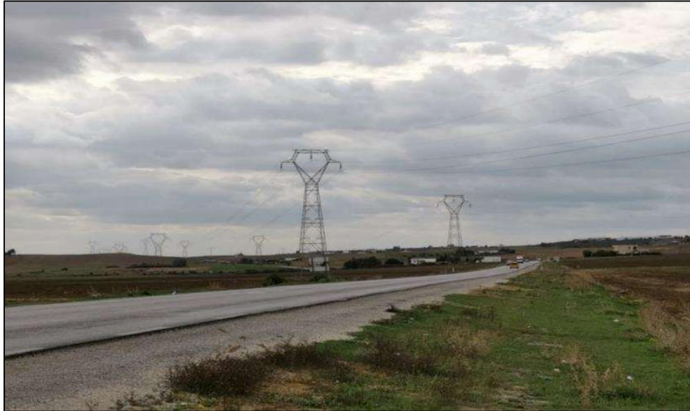
Figure 30 : The two 90 KV power lines between Menzel Temime, Korba and Grombalia
