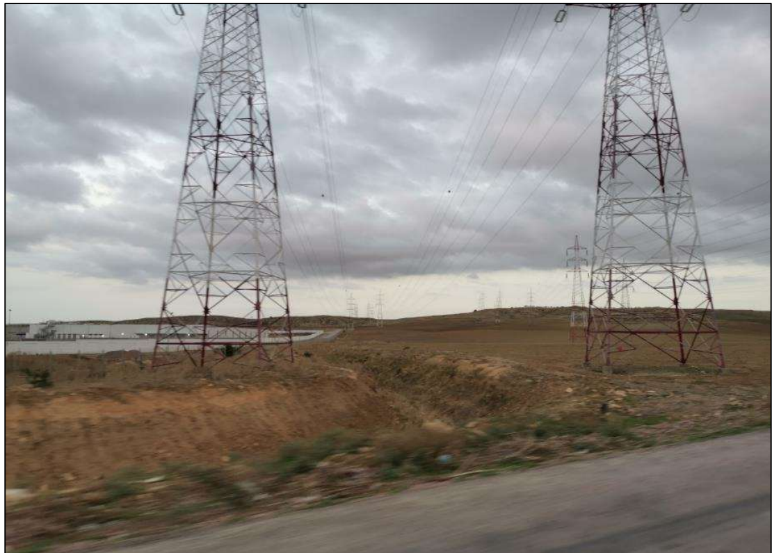
Figure 64 : Existing HV power lines in the area
