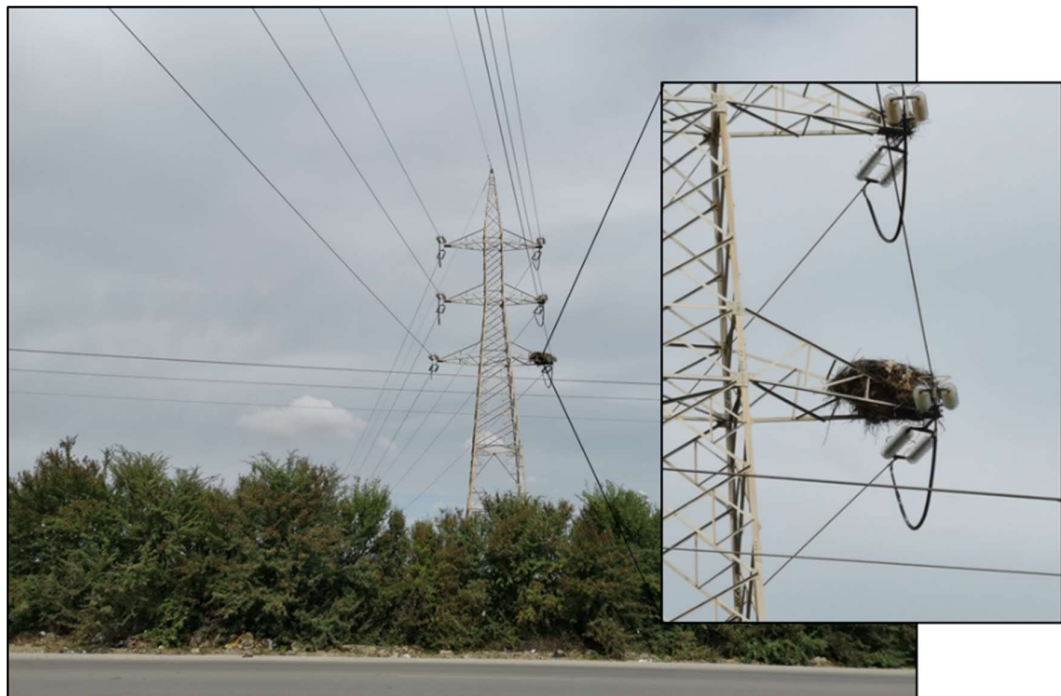
Figure 51 : An OHL power line close to the proposed line route of Mlâabi Mornaguia, As we can see a mitigation measure by adding perches to electricity pylons in order to reduce electrocution for birds (a nesting support for Storks) (36°36'44.09"N, 10°31'34.76"E)
