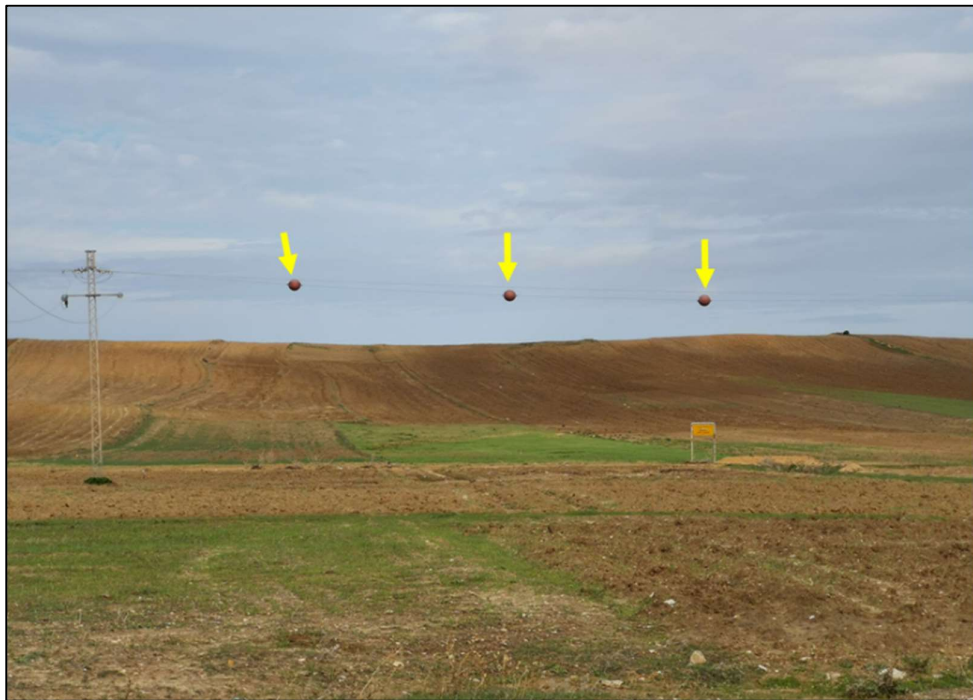
Figure 36 : Protection markers on an MV line near the line route proposed for the Mlâabi-Mornaguia project
